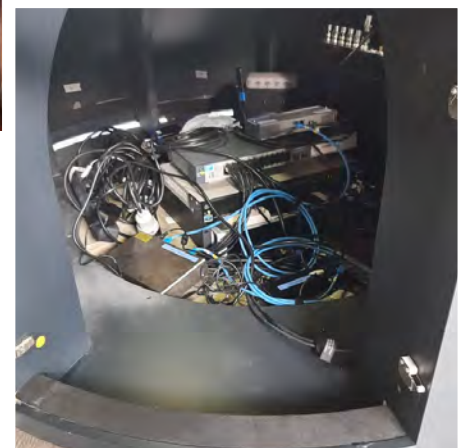
Installations in conference table
